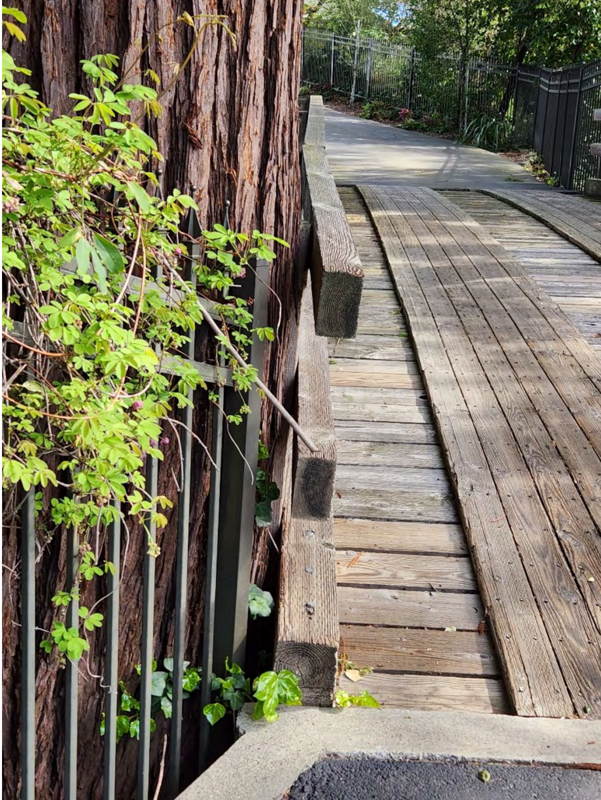
The trunk of the tree is already pushing against the wooden railing along the bridge. Structural damage will likely occur as the tree continues to enlarge.
